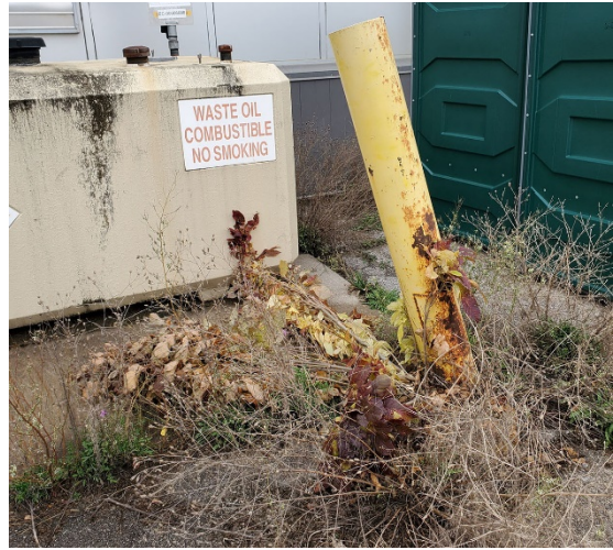
Bollards worked but required repair. Cut weeds around bollards (in summer, will hide bollard).
