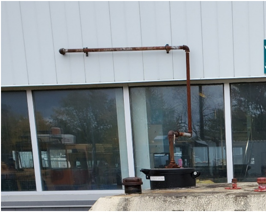
Aboveground lines only. Waste oil comes in from building. Some surface rust – no apparent major damage. RPOps does annual corrosion testing.
