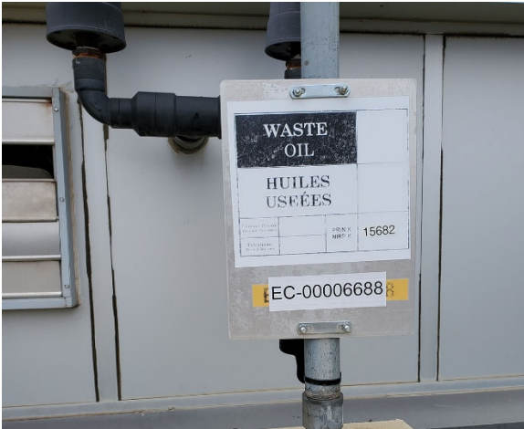
Tank identified by signage (EC) and K-Prin.
