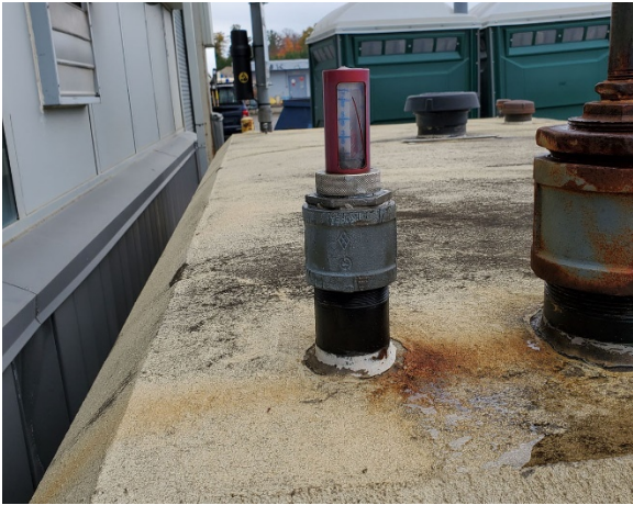
Level meter is readable and functional.
