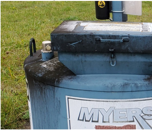
Level meter unreadable. Replace or have dipstick for readings.
