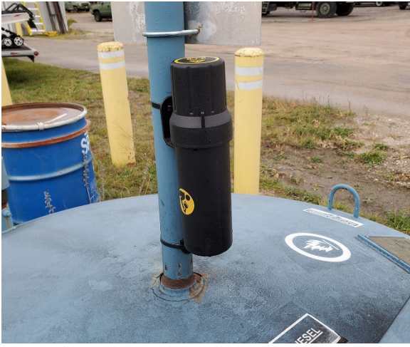
EP receptacle is present.
