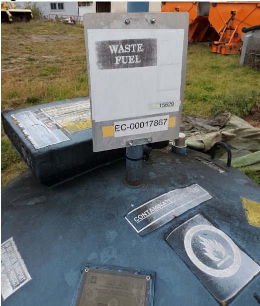
Tank identified by signage (EC) and K-Prin.
