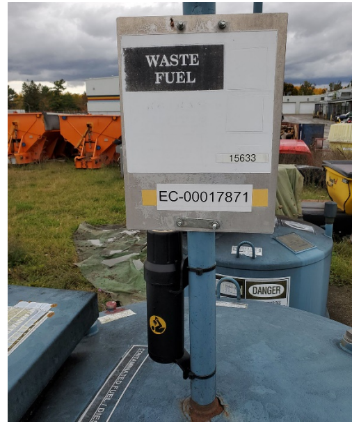
Tank identified by signage (EC) and K-Prin.
