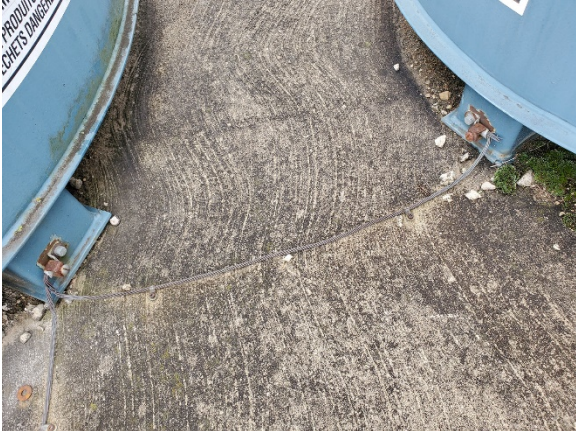
Gas and diesel tanks have grounding wire.
