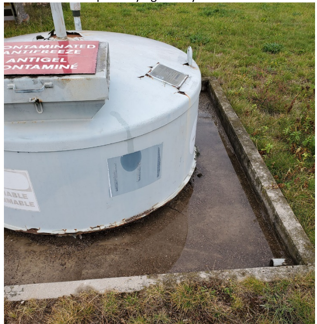
Tank is below grade and filled curbs are concrete is filled with water; no place to drain out; possibility of oily-water spill.
