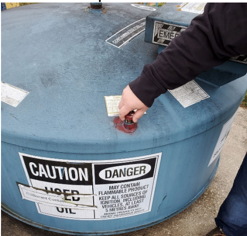
Dipstick for leak detection present.
