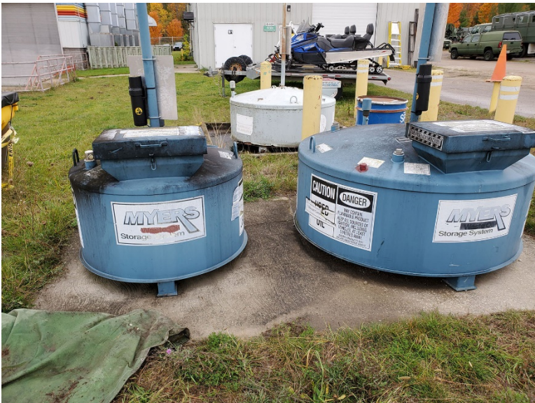
Blackened tanks – likely from exhaust from vehicles parked near the tanks: demonstrates vehicles have been parked close by.
