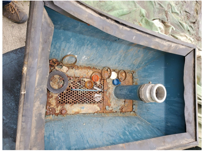
Minor items in spill box. Remove and dispose.
