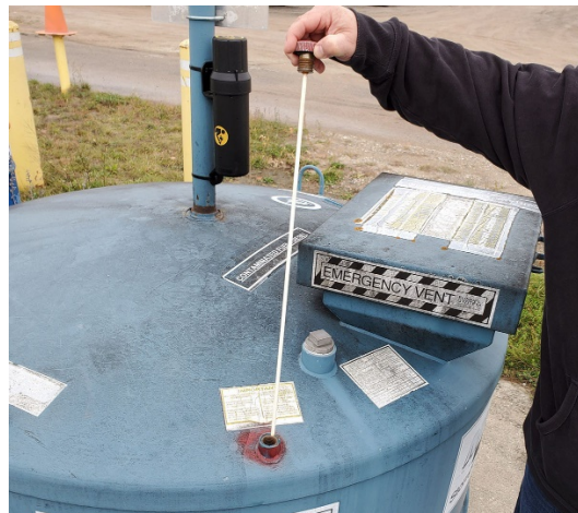
Dipstick reading is EMPTY.
