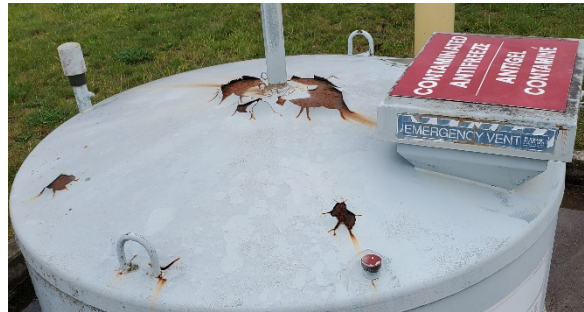
No level meter on the tank.
