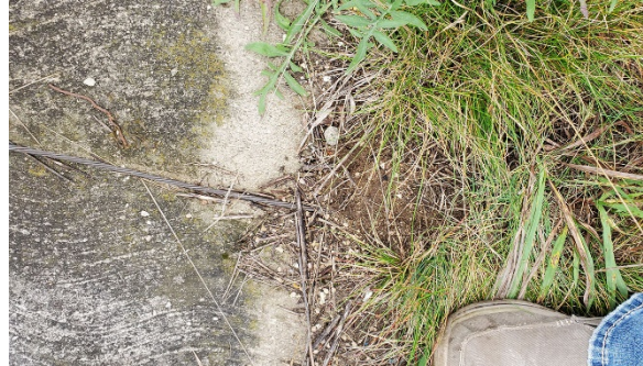
Grounding wire attached to grounding post for gas and diesel tanks.
