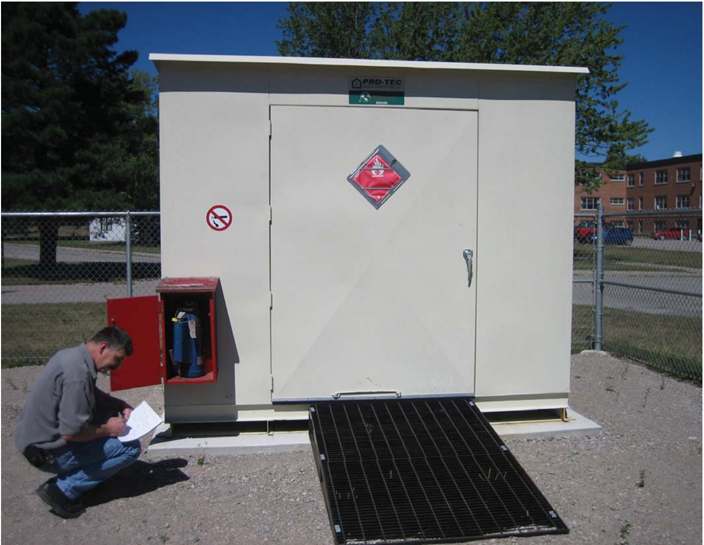
Storage areas must be appropriately sited and include adequate secondary containment, appropriate placarding, regularly inspected fire fighting equipment, grounding, and suitability to the products it contains.
